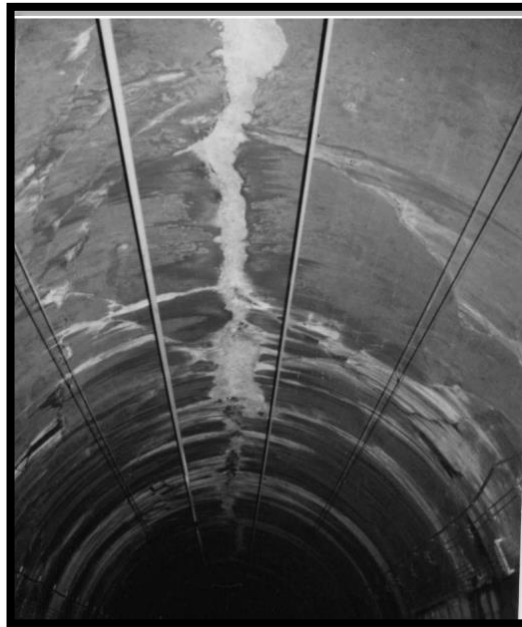
Figure 2.2: Compressive failure caused a longitudinal crack line in the Tsukayama Tunnel (Sources: Asakura & Kojima, 2003)
