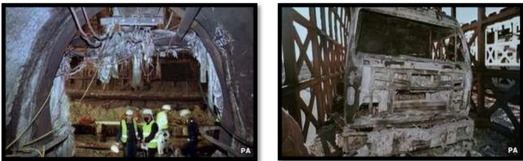
Figure 2.1: The infrastructure of Channel Tunnel was damaged and a fire on a truck caused a great deal of damage during 2008 fire incident (Sources: Carvel, 2010)
