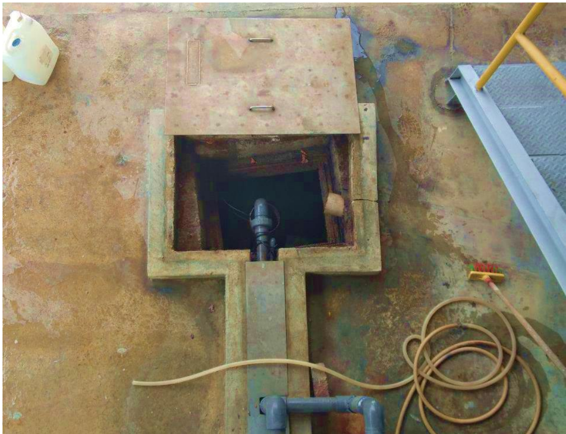
Figure 3.2: Influent stage of treatment plant.
