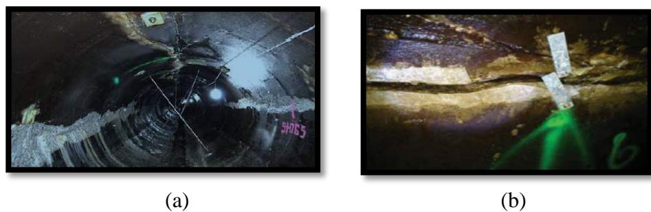
Figure 2.2: Pucara Headrace Tunnel (a) stretch of damaged and (b) fracture detail
