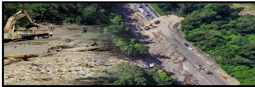
Figure 2.5: Landslide at Kuala Lumpur-Karak Expressway.
