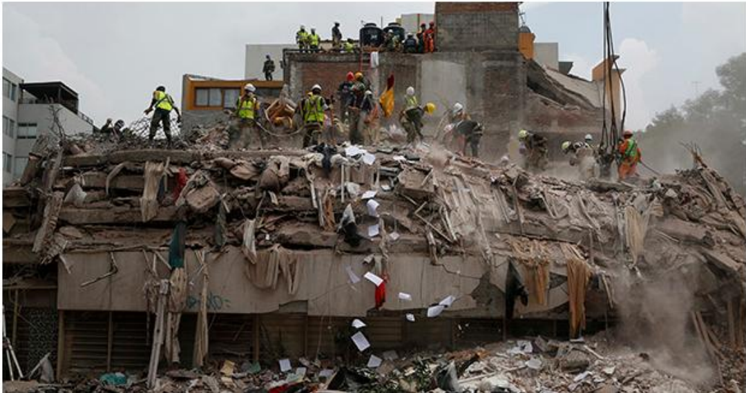
Figure 1.1: Mexico City building collapsed with 7.1 magnitude earthquake ( https://finance-commerce.com/2017/09/mexico-assesses-quake-damage-to-economy/ )
