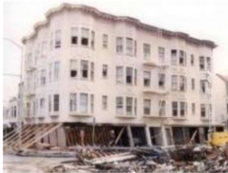
Figure 2.3: Collapse of multi-storey building due to soft storey. (Nirkhe et al., 2016)
