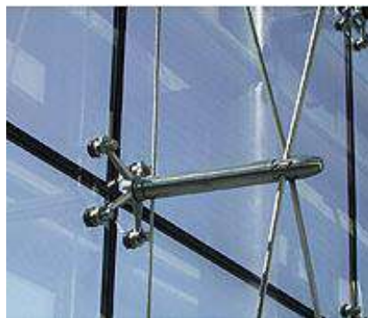
Figure 2.14: Point-fixed bolted glass system using a spider fitting and perforated glass (ArchitectureWeek, 2011)
