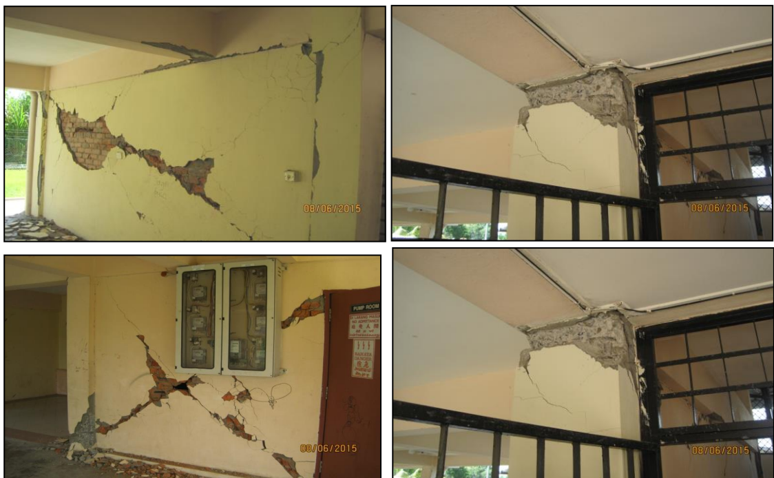
Figure 1.2: Structural Damages of Ranau Hospital
