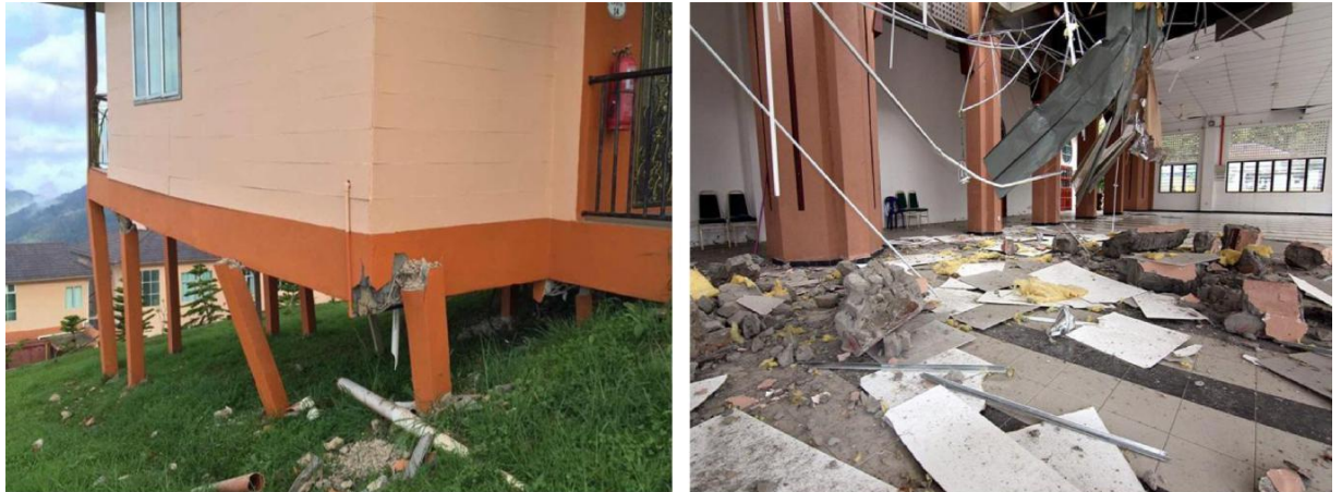
Figure 2.3: Damages from Ranau earthquake (Awani, 2015)
