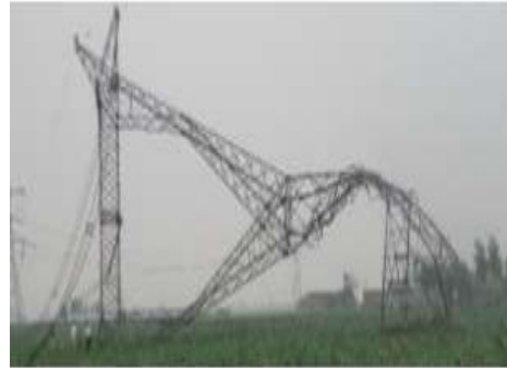
Figure 1.2: 500 kV transmission tower collapsed during severe storm (Cai et al., 2014).
