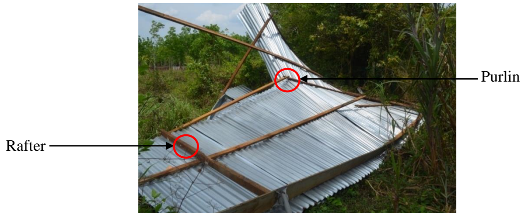
Figure 1.2: Total roof blown-off
