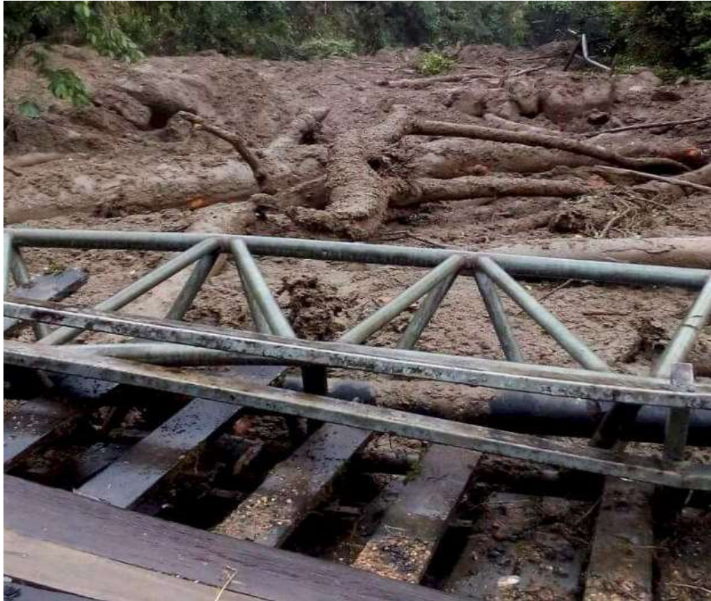
Figure 1.2: Destruction of Bridge Caused by Mudflow at Ranau (Sario and Lee, 2015)
