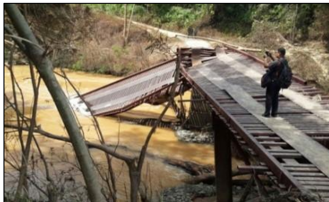
Figure 1.3: The Partially Collapse of Aur Gading Bridges in Pahang (Astroawani, 2015)
