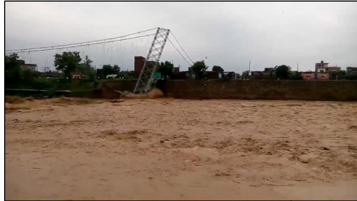
Figure 1.5: The Collapse of the Suspension Bridge due to the Flash Flood (The Telegraph, 2016)
