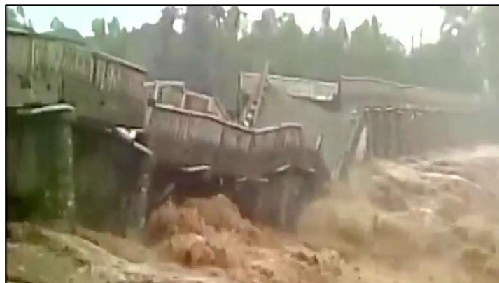
Figure 1.6: The Bridge Collapsed in Heavy Rain in Kangra District of Himachal Pradesh on 11 August 2016 (Newscrunch, 2016)
