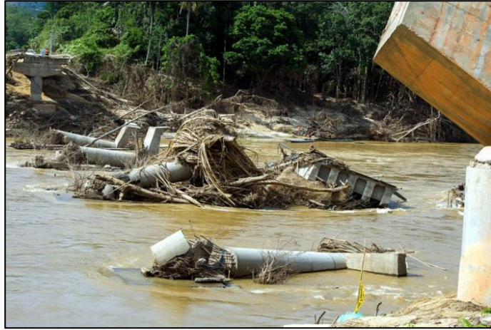
Figure 1.1: Wash Away of the Decks of Pulau Setelu Bridge in Kelantan (Thestar, 2015)
