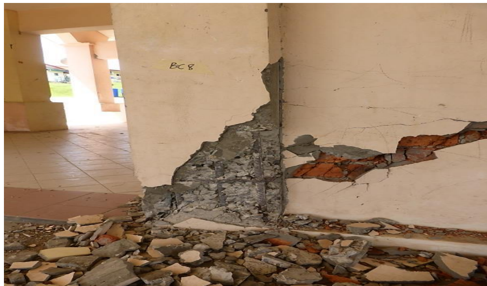
Figure 1.2 : The crack at the bottom of column at Hospital Ranau
