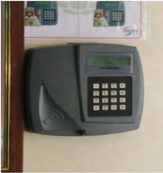
Figure 2.7: Centralized Access Control System (in front of Computer lab)
