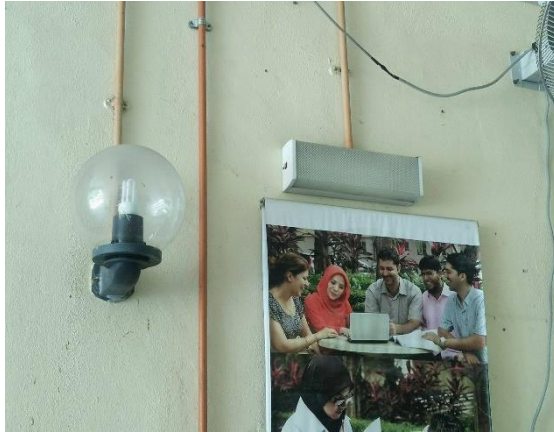
Figure 2.4: Emergency lamp (at structure lab)
