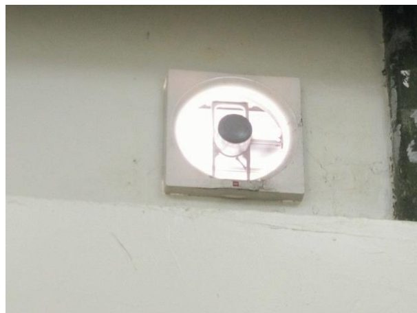
Figure 2.6: Extract Fan (at hydraulics lab)
