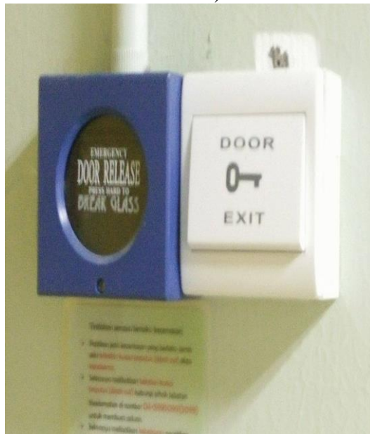
Figure 2.10: Emergency Door Release (inside Tutorial Room)
