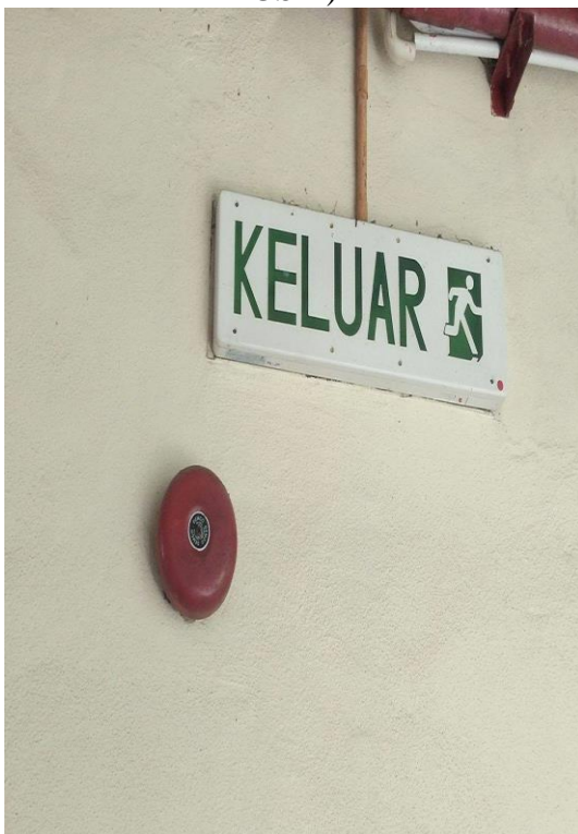
Figure 2.14: Exit Sign (at Structure Lab)
