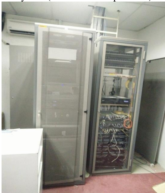
Figure 2.9: CCTV Control Room (inside Computer Lab)
