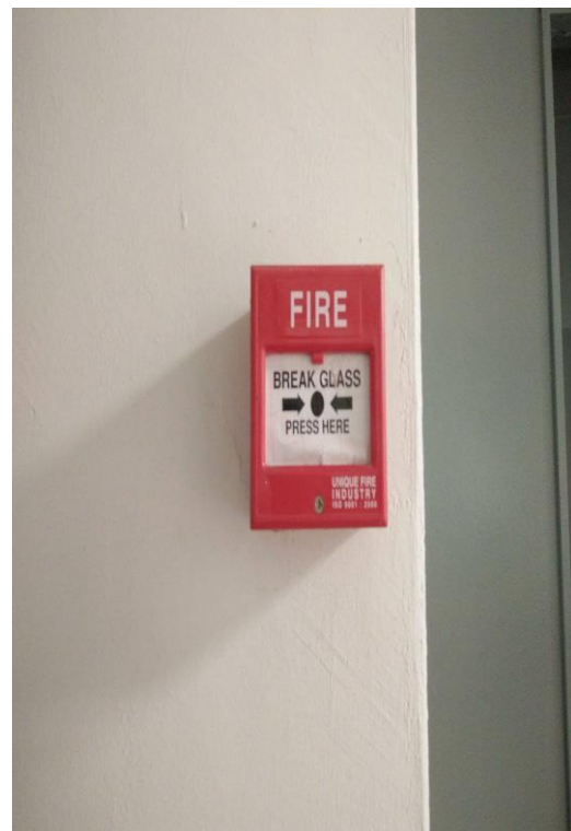
Figure 2.15: Fire Alarm System (at Tutorial Room walkway)
