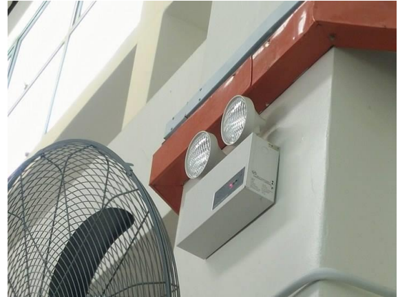
Figure 2.5: Emergency lamp (at hydraulic lab)
