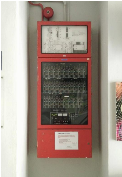
Figure 2.12: Fire Control Panel (in front of the School of Civil Engineering, USM)
