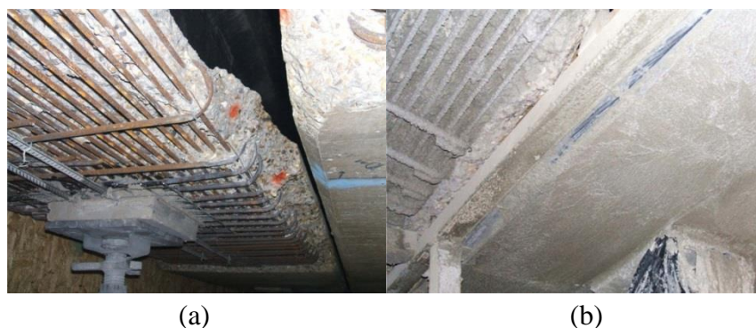
Figure 2.5 Before (a) and after (b) photo of Dean's Brook Viaduct repair work (Wheatley et al., 2014)
