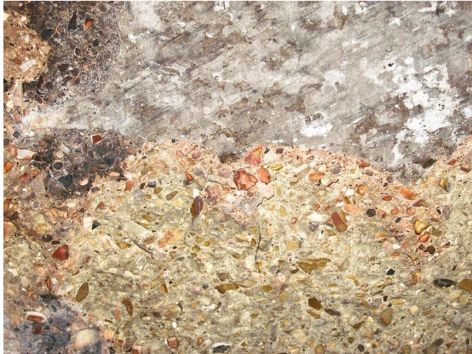
Figure 2.2 Concrete spalled from slab soffit showing pink/red discoloration (Rogerson, 2017)
