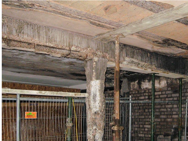
Figure 1.1 Spalling of concrete to beam and a column caused by fire
