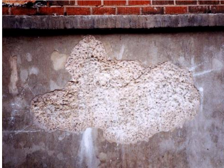
Figure 2.3 Concrete spalling on wall (Rogerson,2017)
