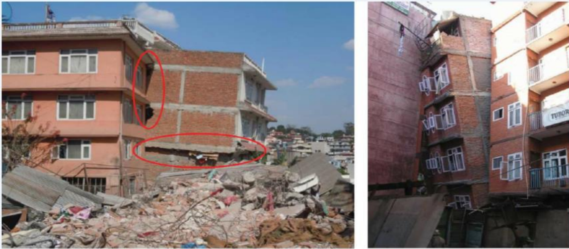
Figure 1.1: Collapse of intermediate stories due to pounding of adjacent buildings (Rai et al., 2016)
