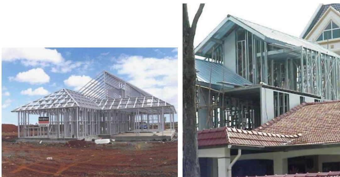
Figure 1.1: Example of structural framing system using light gauge material for residential building (Authority, 2003)
