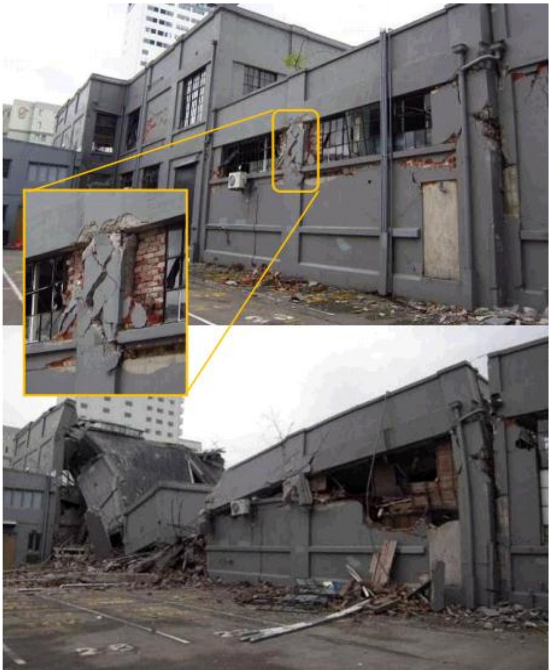
Figure 1.5: Effect of local behaviour of structural member on global response of RC frame (Kam et al., 2011)
