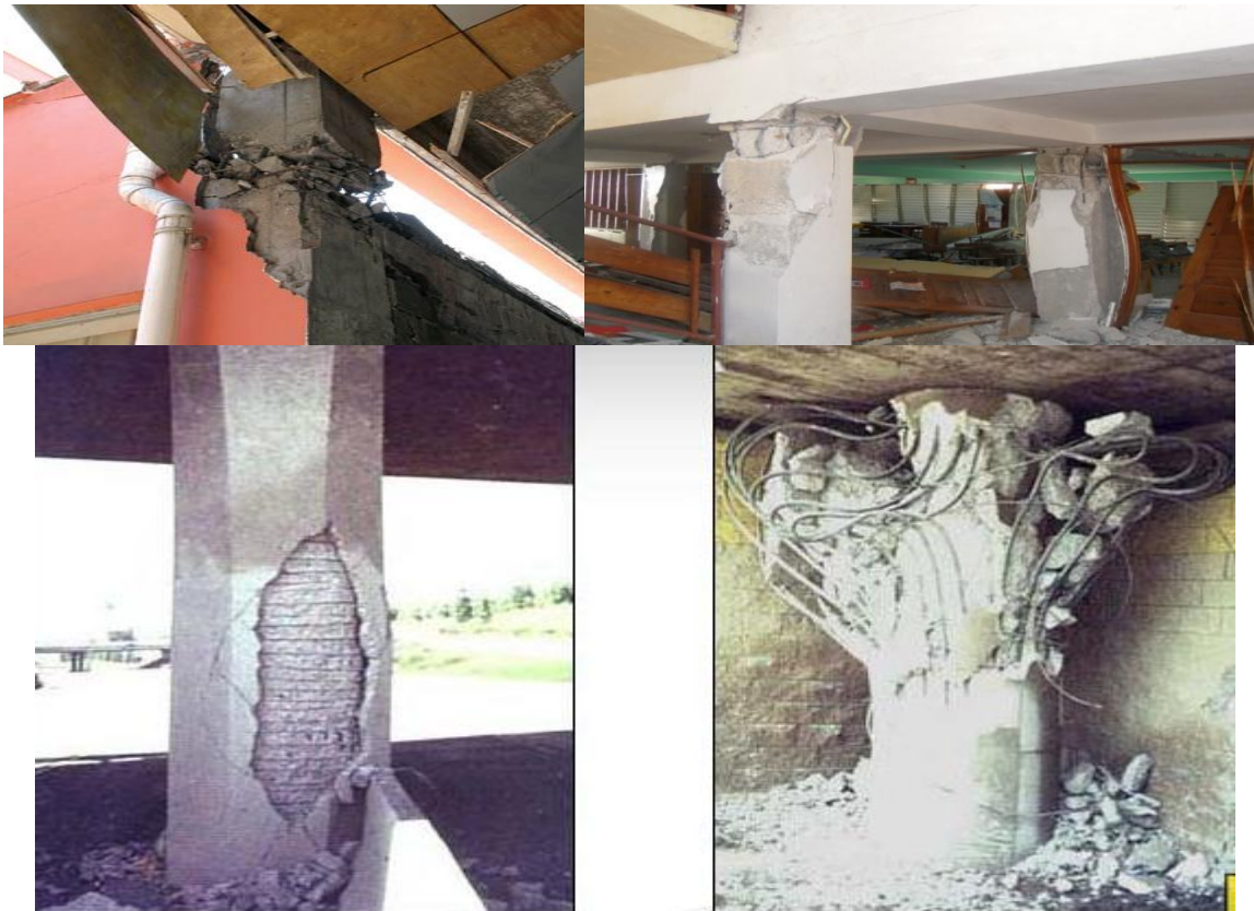
Figure 1.1: Failure of RC columns due to earthquake (Canfield and Sabrina, 2010)
