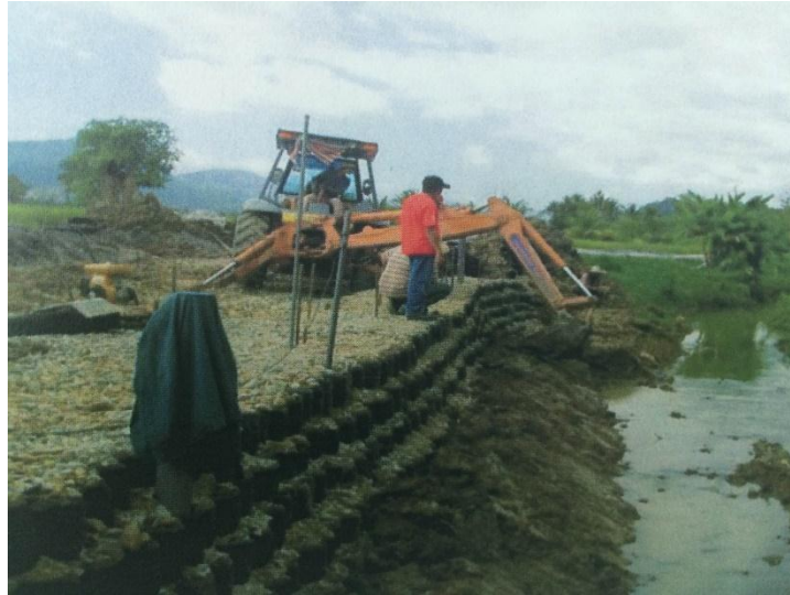
Figure 1.2: Construction of 8R mat system for slope stabilization and erosion control (Safari, 2012)
