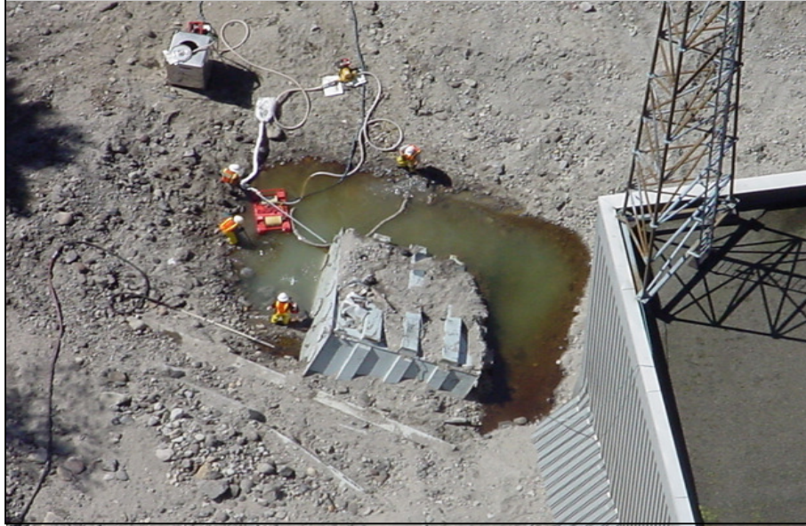
Figure 2.6: Cleanup workers removing the oil from transformer below the damaged power house in Southwest Washington, U.S in 2002 (Washington State Department of Ecology, 2002)
