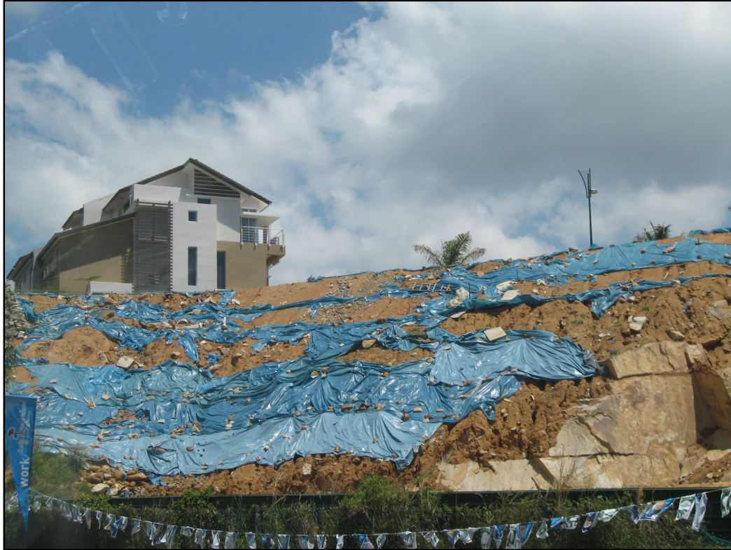
Plate 1.1: Typical example of Soil Erosion features on construction site
