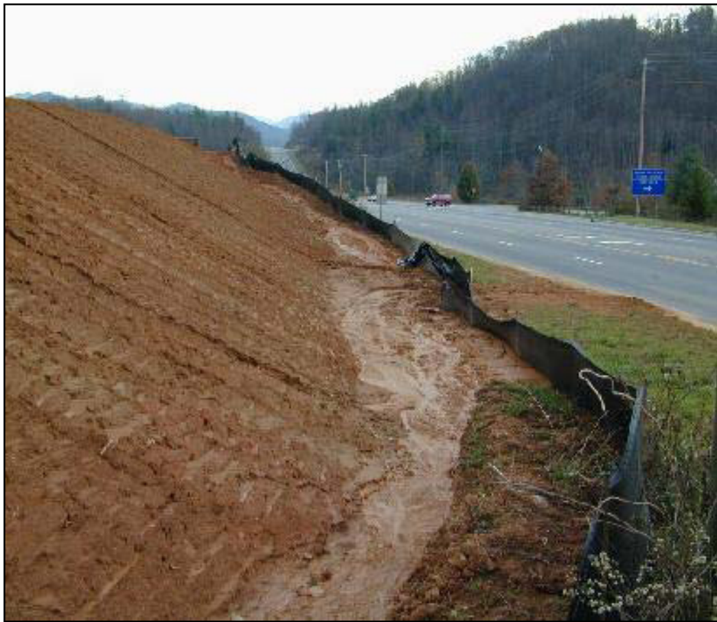
Plate 2.1: Soil erosion phenomena on bare slope
