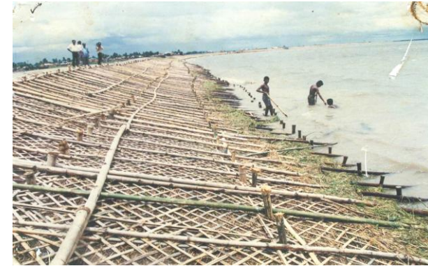
Figure 5. Protection of slope by locally available Chala grass encased in a bamboo split frame
