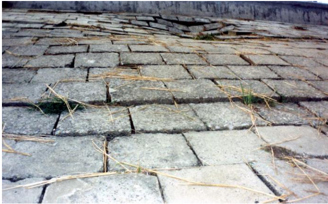
Figure 8. A view of the CC block settlement in the upper part of the slope during the 2003 flood (second damage)
