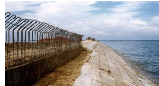
Figure 13. Construction of RCC guard wall with earth filling that was not compacted
