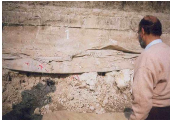
Figure 11. Cavities below geotextiles
