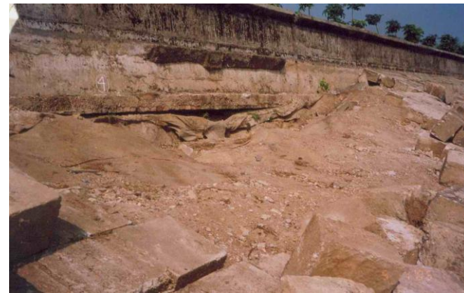
Figure 9. One of the breaches at the bottom of the guard wall approximately at the middle of the embankment
