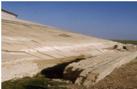
Figure 6. Brick toe wall collapsed (under water) and CC blocks slid down slope (view in dry season, first damage)
