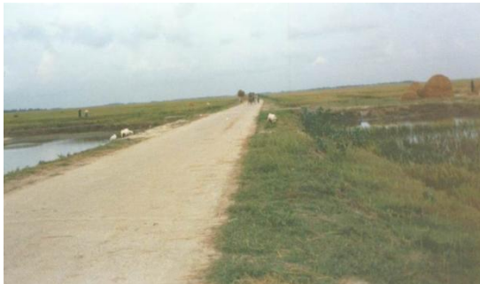
Figure 3. Submersible concrete road (low) dykes in the haor area to prevent early flash floods
