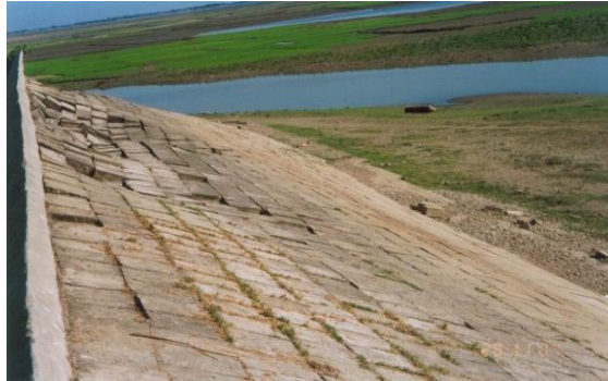
Figure 10. Settlement of CC-blocks the crest of the guard wall during storm wave during 17 th August, 2004
