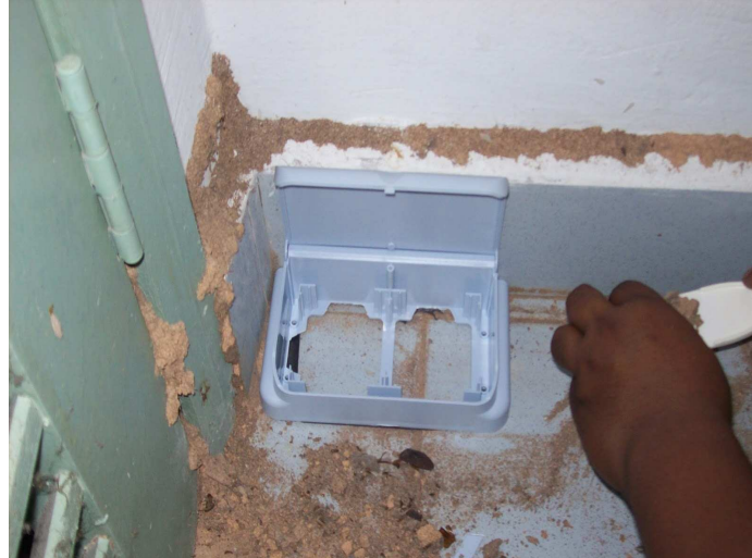
Figure 3. Serious termite attacks ondoor frames
