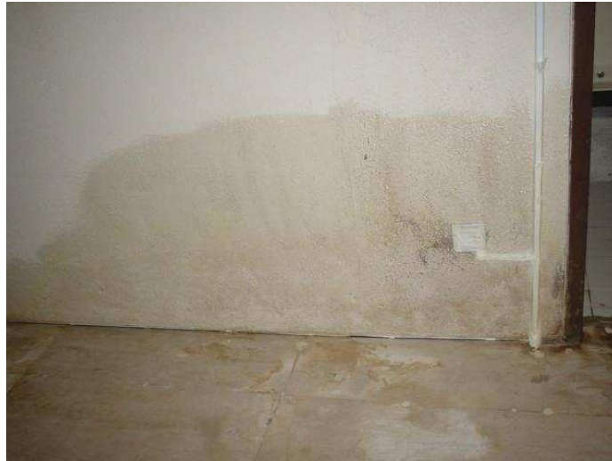
Figure 2. Dampness on wall section
