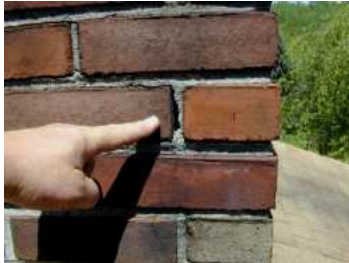
Figure 1. Problem of worn mortar joints
