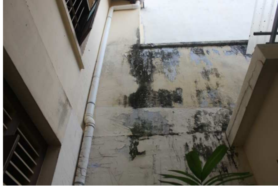
Figure 7. Penetrating damp evidence
