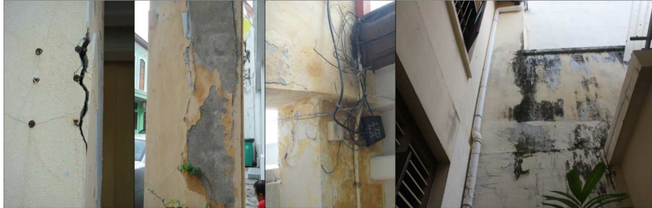
Figure 2. From left: the paint layer was peeling. Second: there is crack on upper part of column. Third: There is colour change, Right: effect from dampness
