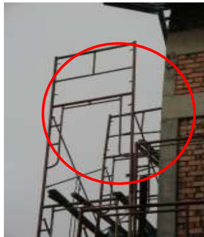
Figure 2 : No ledgers and loose of scaffolds components at Bungalow Project.
