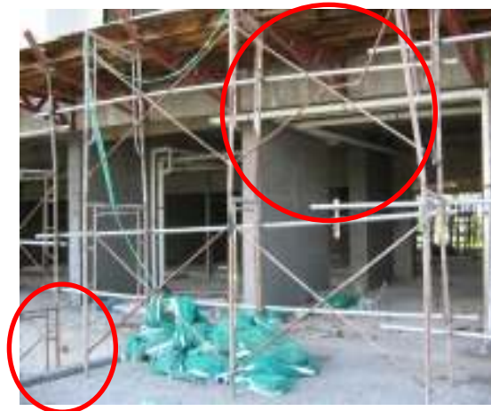
Figure 3 :Some of the cross bracing are bent and no base plates at Apartment Project
