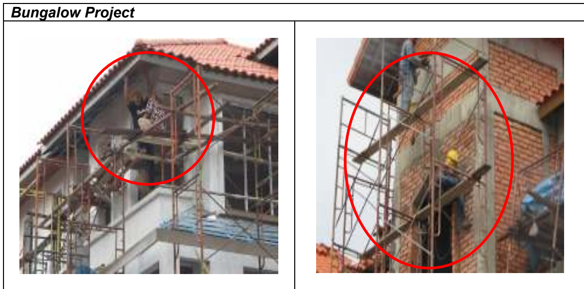
Figure 4 : Construction workers done their jobs above 3meter on incomplete scaffolds that without guardrail systems and fall protection equipments.
