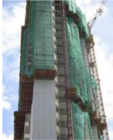
Figure 5 : Complete with safety net and overhead protection at Apartment Project to prevent any injuries or accident.
