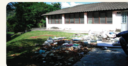
Initial cleaning by the Development Office of the Eco Hub began on Saturday 17 January 2009. Two days later on Monday, the Eco USM Team had already moved into the building
