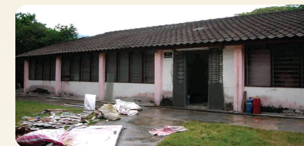
General repair and restoration work at B11 (the Eco Hub) starting from 2 December 2008
