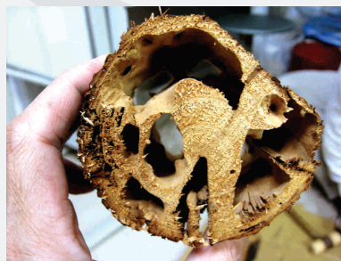
Figure 4: Damage by drywood termites.
