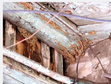
Figure 5: Damage by subterranean termites.
