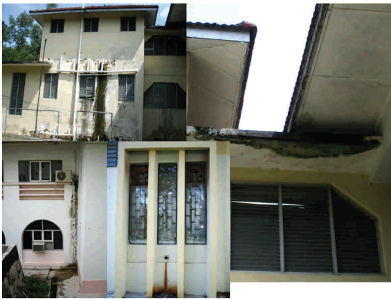
Figure 33: Poor moisture management is one of the most important factors contributing to termite infestation in buildings and structures in USM Minden campus.
