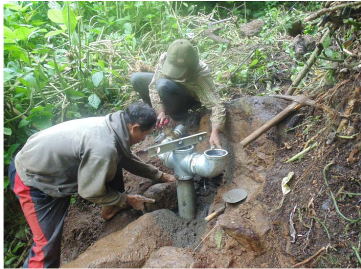
Picture 3) The villagers plant hydram pipe to bring up water level from the water source. With this technique, the villagers can obtain clean water. Before, the villagers had to walk for around 2 km down the hill to get the clean water
