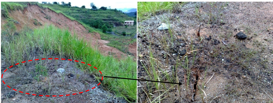
Photo 1: Small fractures located at the collapsed area in Selangor.
