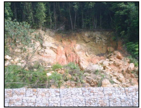
Figure(5.4): General view of Jalan Tun Sadron slope
