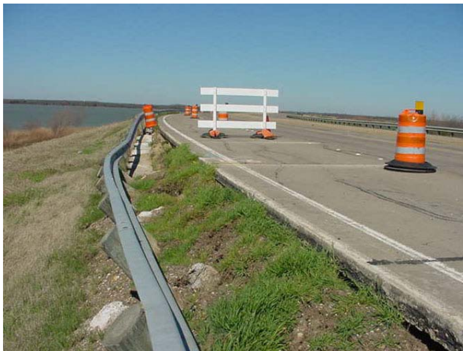
Figure 2.5: Initial slope failure along the roadway (Gregory, 2006)
