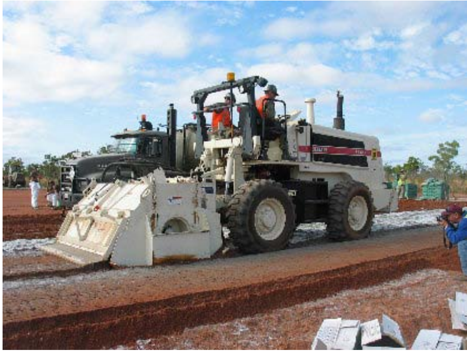
Figure 2.3: Fibre and cement mixed using slow speed Terex (Joint Rapid Airfield Construction, 2007)
